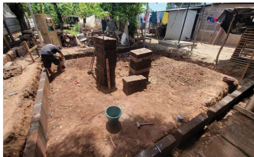
A community worker begins laying the foundation for a new home in El Platanal.
