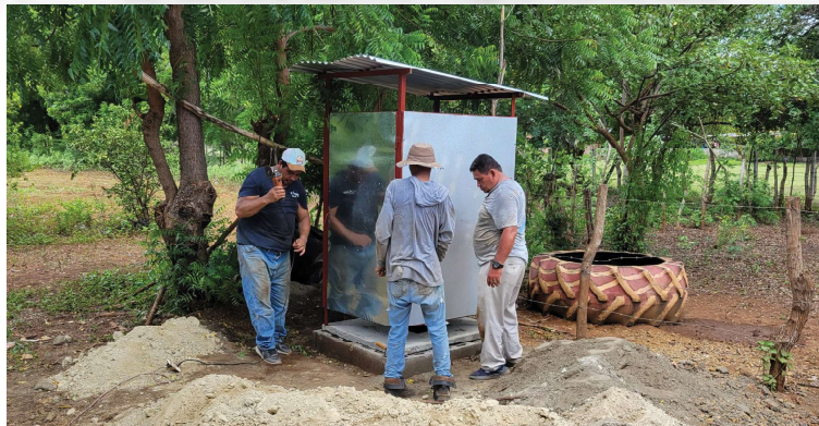
Three community workers stand beside a newly built latrine, part of a project focused on improving sanitation while restoring dignity and opportunity for families.
