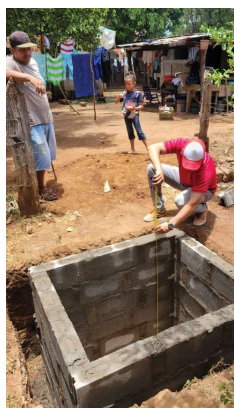
Below - A worker measures the foundation of a latrine under construction, carefully preparing the base before the next stage of building.
